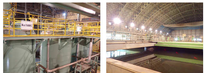
Fig.1(left) Neutralization tanks
