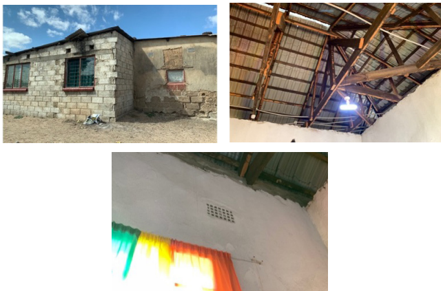
Fig.2 (upper left) Exterior of the building Fig.3 (upper right) Galvanized steel roof Fig.4 (lower) Air ventilation
